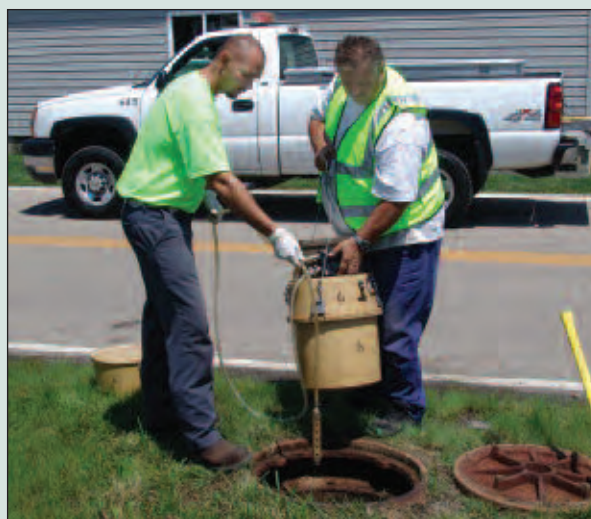
Wastewater Collection System Crew Members Chris Croucher, left, and Kim Campbell install an industrial waste sampler. The device takes readings every 15 minutes to analyze materials in wastewater flows.
