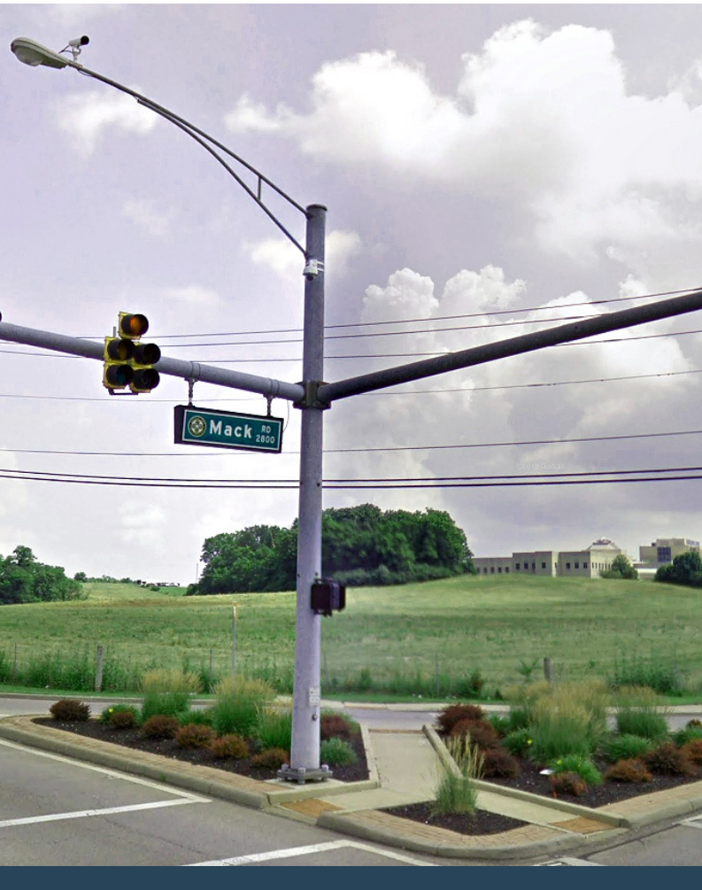
Traffic control and monitoring at Mack and South Gilmore Roads
