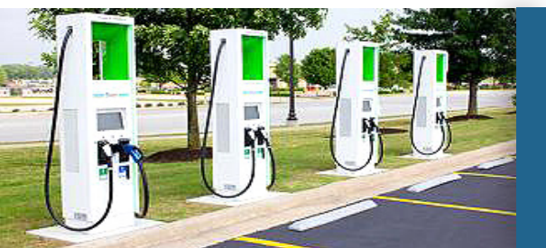
Electric vehicle charging stations
